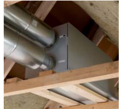
HCH installed in an attic.
